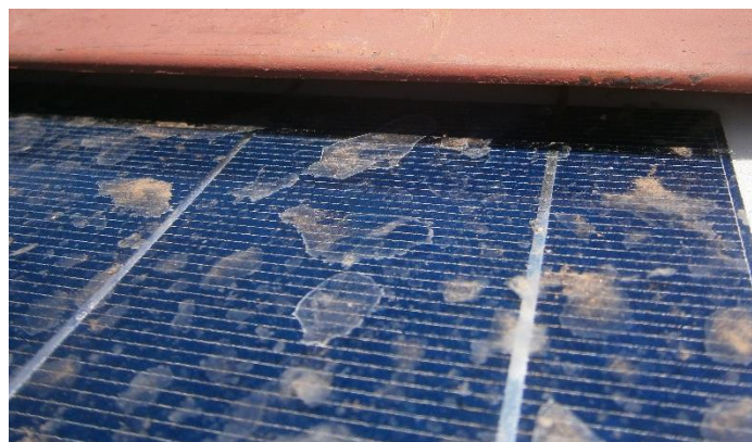
Figure 15: Partially shaded, dirty PV modules in the Northern Highlands, Tanzania. April 2019.
